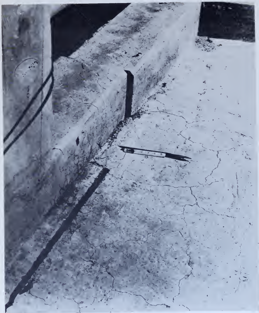
Figure 4.—Typical pattern cracking on the exposed surface of concrete affected by alkali-aggregate action. PX-D-32049.
